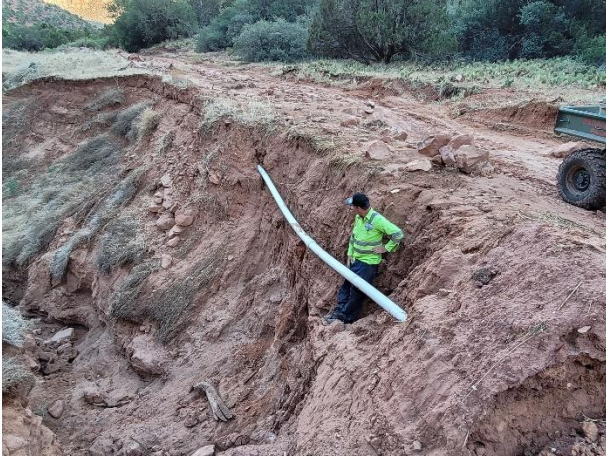
Nathan inspecting another washout in Maxwell Canyon
