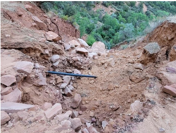
A third washout in Maxwell Canyon, where the pipeline is exposed.
